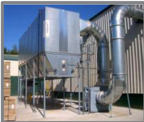
Installed dust removal system.
