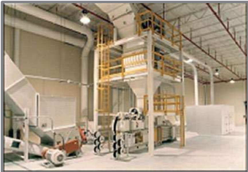
Installed paper trim removal system with dust-shrouded separator inside the plant. Note the box structure beyond the separator, which is a sound enclosure that houses the material handling fans.
