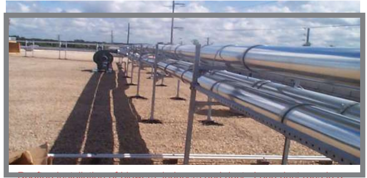
Rooftop installation of blowers, inducers and dust collectors. Long duct runs in a pneumatic system require precise design and engineering to maintain optimal material air flow.
