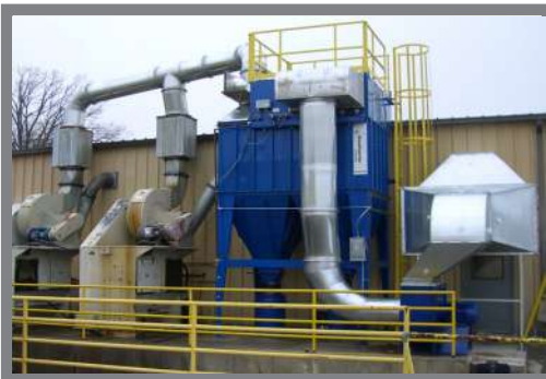
Installed dust removal system.
