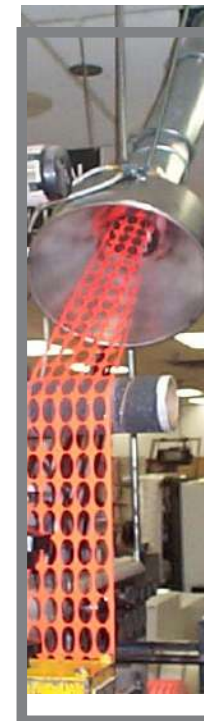
PSA Label Matrix entering the intake at the start of the waste removal system.
