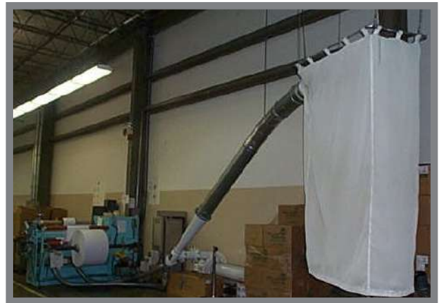
Rented Blower system conveying package for paper trim conveying.
